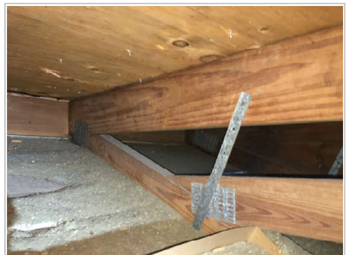
Toe Nail - Not Meeting Nail Requirements
